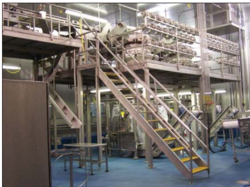
The spiral discharge area has a fine filtration and inspection area. In addition, the radial scale and baggers are supported by a fully welded mezzanine. Source: VCP&A.
