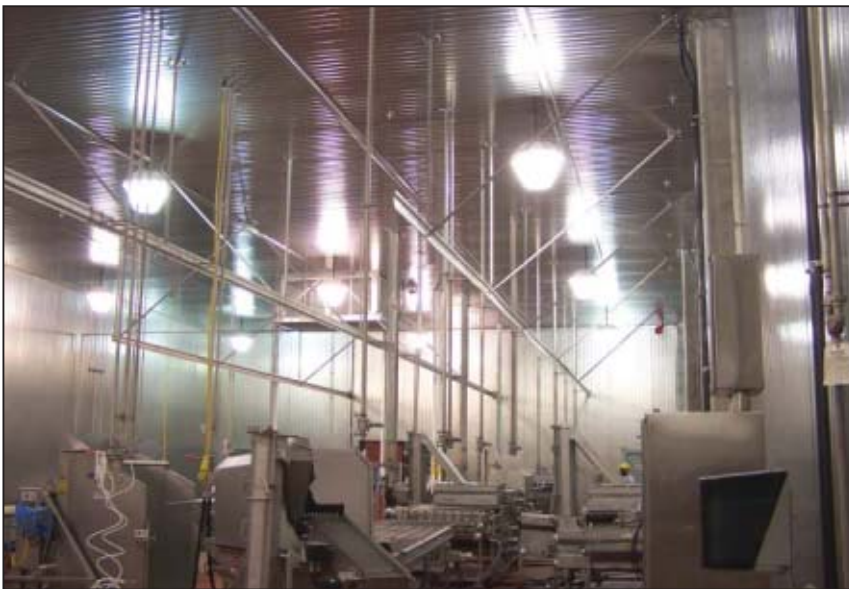
The beginning of the double front-end process uses minimal vertical utility drops while eliminating most horizontal runs. Source: VCP&A.
